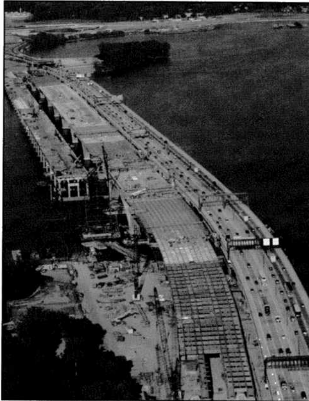
The new 12-lane Woodrow Wilson Bridge replaces a six-lane crossing that produced one of the most notorious bottlenecks in the nation.
