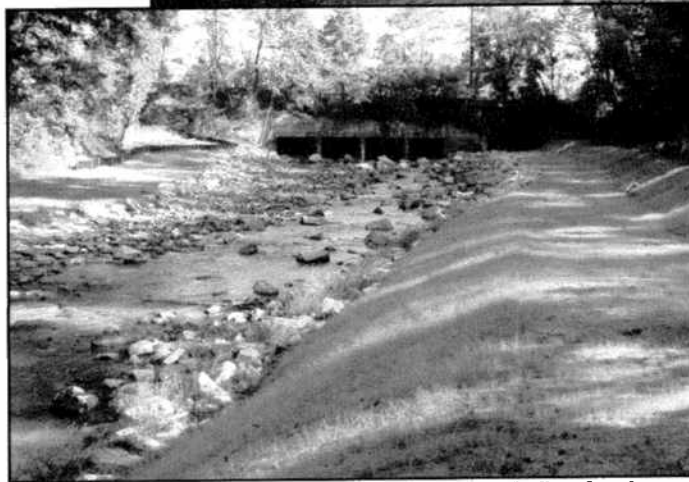
Blockages resulting from erosion and culverts in Indian Creek were addressed with a rock ramp and bank stabilization.
