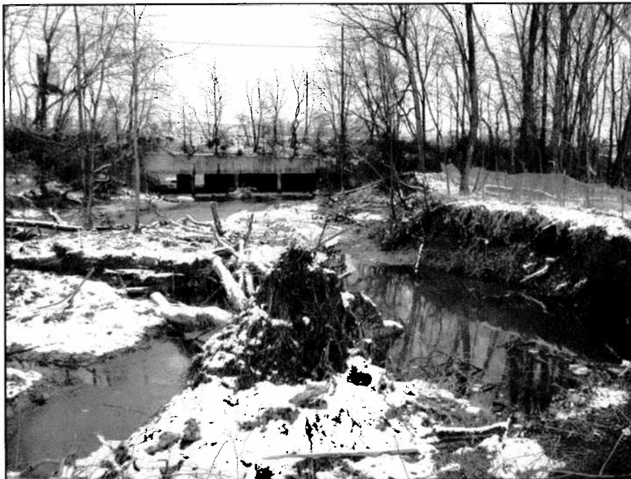
Indian Creek before. Stream corridors suffered from degradation and habitat loss due to erosion and abandoned utility lines, concrete fords, dams and grade control structures.
